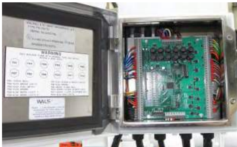
Primary Control Unit [PCU] - internal view Unit is ATEX approved
